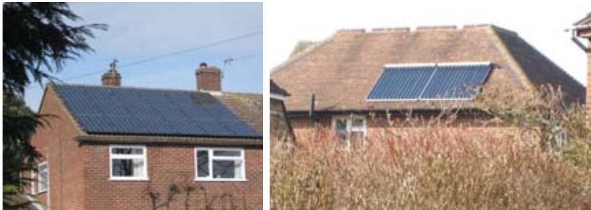
Local examples of photo-voltaic and solar energy panels respectively
